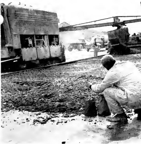
THE SLUMP TEST (FOREGROUND) IS INDICATIVE OF CONSISTENCY AND IS MADE FREQUENTLY AT BOTH LARGE AND SMALL JOBS
